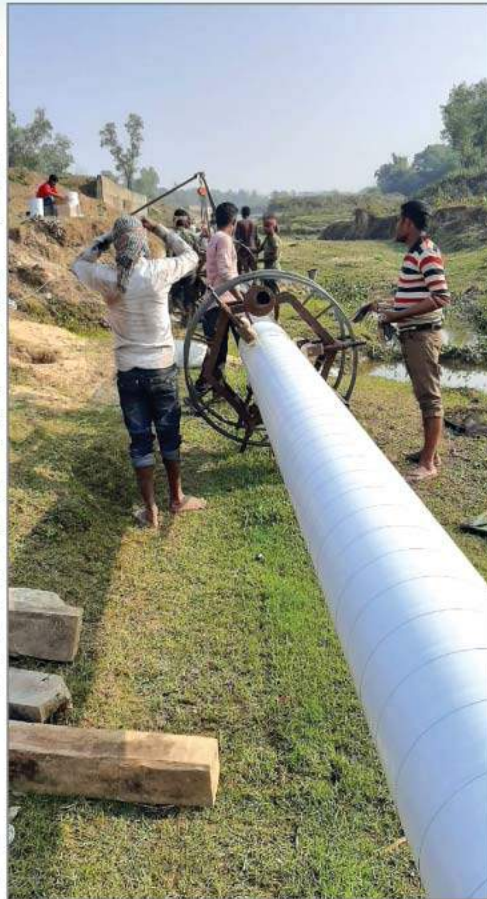
Pipeline construction work for supplying gas to Jamuna Industrial Park, Madhabpur, Habiganj.
