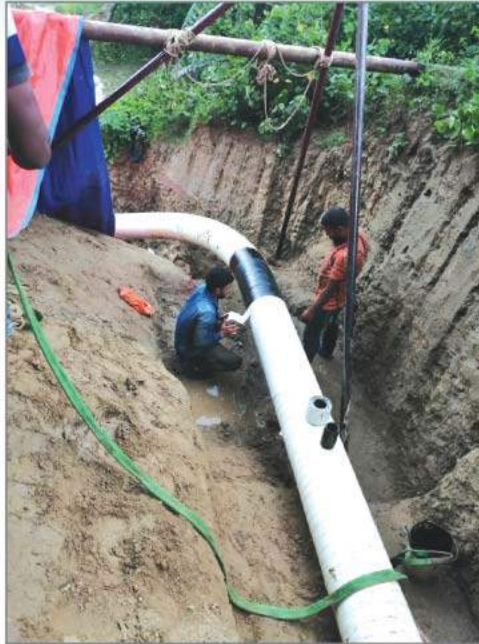
Pipeline construction work for supplying gas to Jamuna Industrial Park, Madhabpur, Habiganj.
