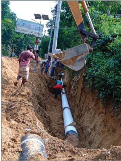
Pipeline construction work for supplying gas to Bangabandhu Sheikh Mujib High-tech Park, Sylhet.
