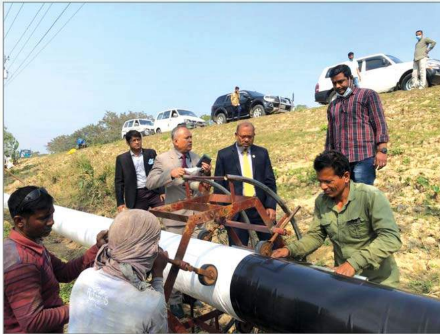
The Managing Director of JGTDSL visiting pipeline construction work to supply gas to Bangabhandhu Sheikh Mujib Hi-Tech Park, Sylhet
